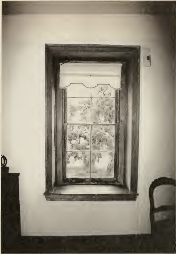
Figure 41. Interior view of north window in second floor northeast room illustrating an example of the type of windows that were installed in the 1820s. (1993.)
